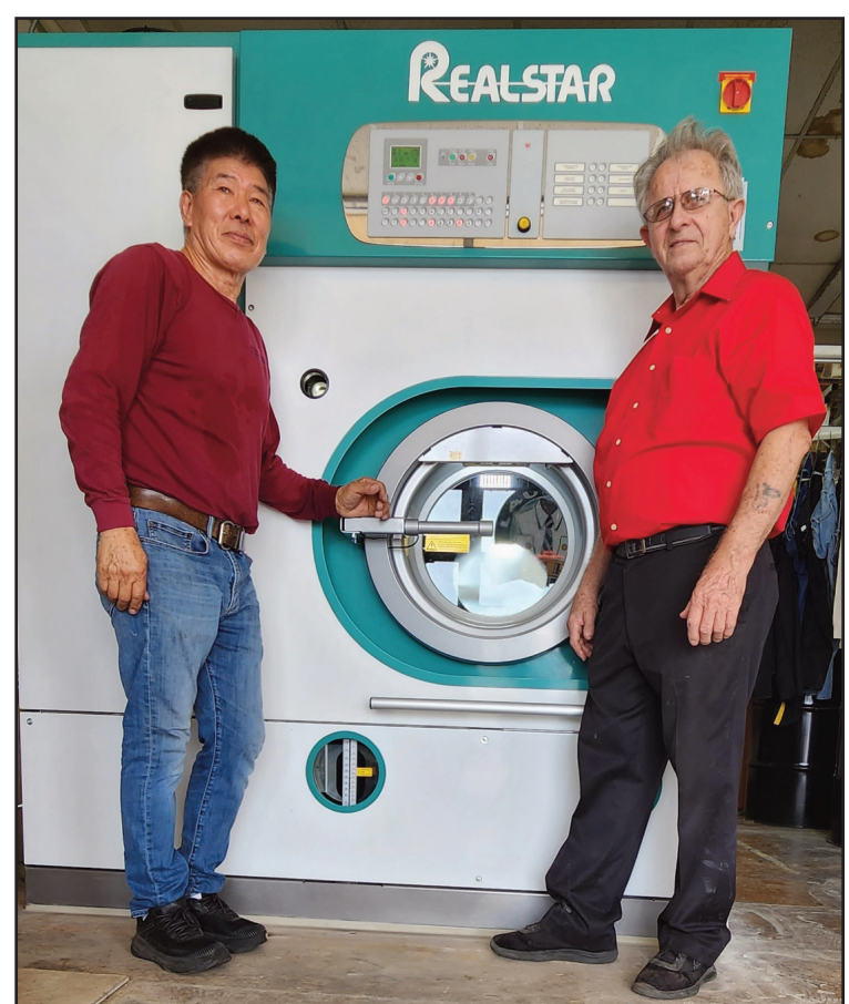
A new REALSTAR KM218-C was purchased and installed by Sun City Cleaners in Sun City, AZ. Pictured at the start-up were Yong Pak (left) of JP Trading and Don Clayborn, owner of Sun City Cleaners.
